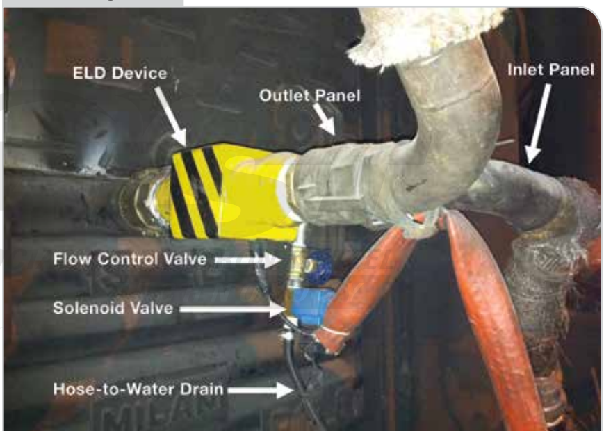
New leak detection device installed on the water-cooled panel of an operational EAF to perform the ELD Technology tests.
